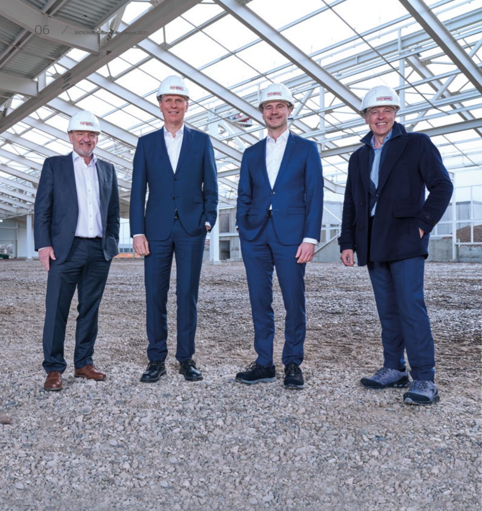
RATIONAL's Executive Board inspecting the progress of construction work in Wittenheim at the beginning of February 2022.
